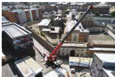
Cobalt's CT and MRI units being craned into position in the heart of Gloucester, as part of the new Quayside Community Diagnostic Centre.
